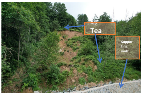
Figure 2. A translational debris flow in the tea plant garden that overflowed the paved road near the Sirtoba village, Arhavi, Türkiye (Photo by M.Yavuz 2023)
